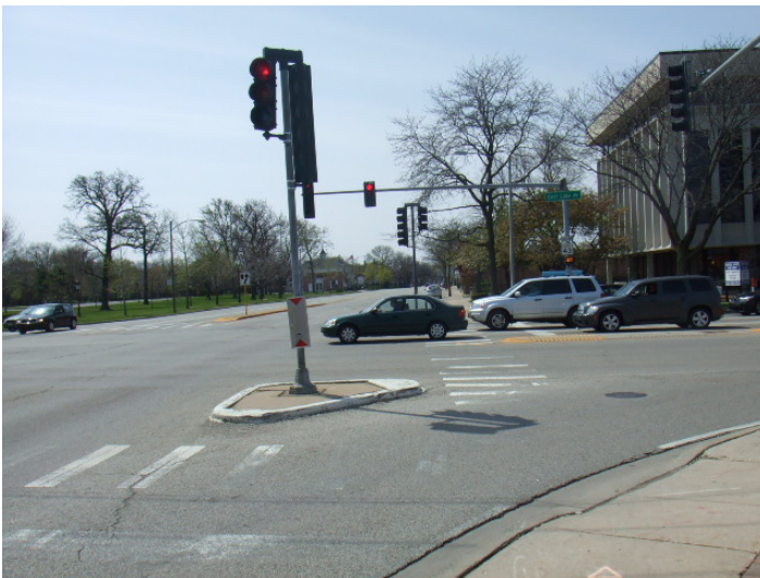
Inadequate pedestrian refuge. Bank of America looking south along Waukegan towards Lake.
