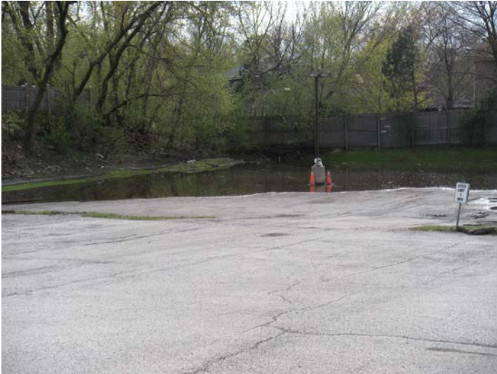
Inadequate drainage. Behind Loren Hyundai.
