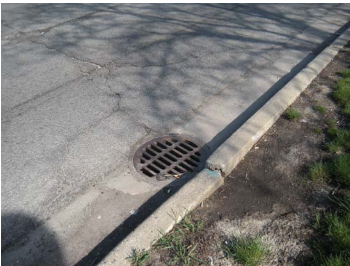
Aging infrastructure. Waukegan adjacent to Staples shopping center.
