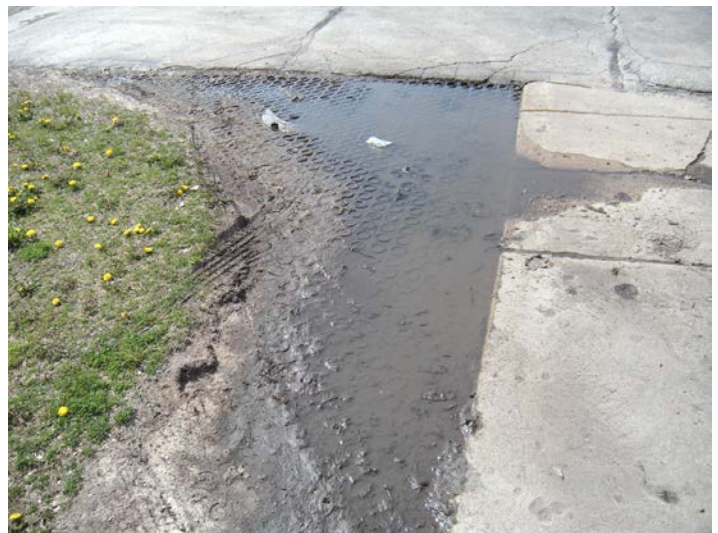
Impervious paving not working. Expo 2000 driveway.
