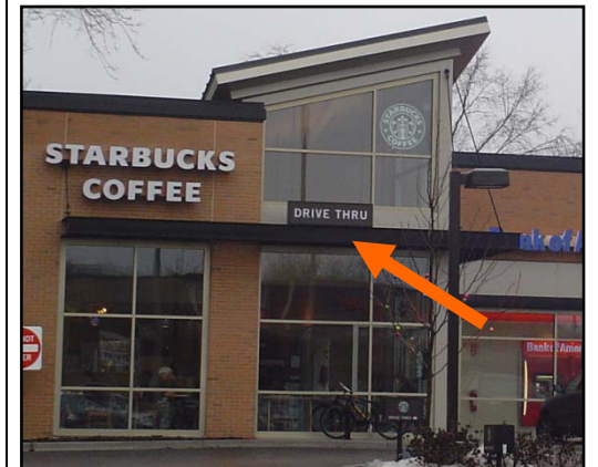
A box sign is not integrated with the canopy (5d)
