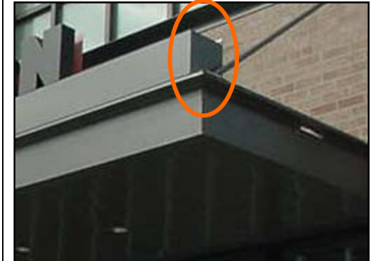
The raceway has not been concealed behind or designed as part of the canopy (5c)
