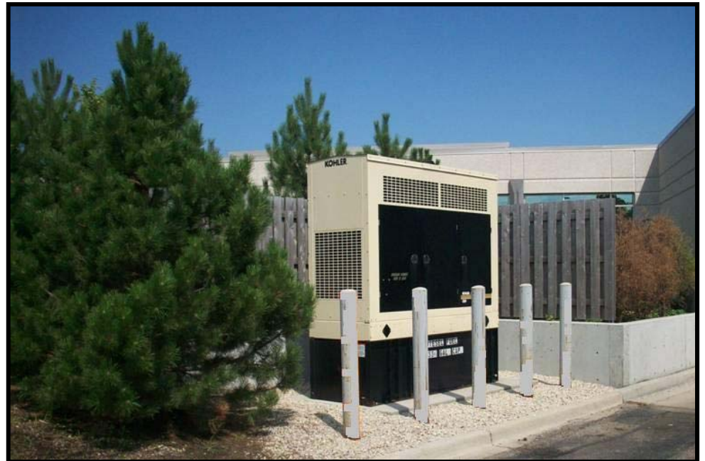
A good example of mechanical equipment being screened year-round by evergreen plantings and solid fencing. It is protected from vehicles by concrete bollards and vents away from the landscaping to protect the plants.
