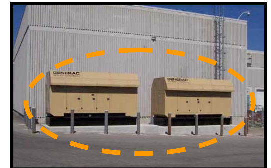
(1). Use of a screening wall in a similar color to the façade would better screen the generator.
