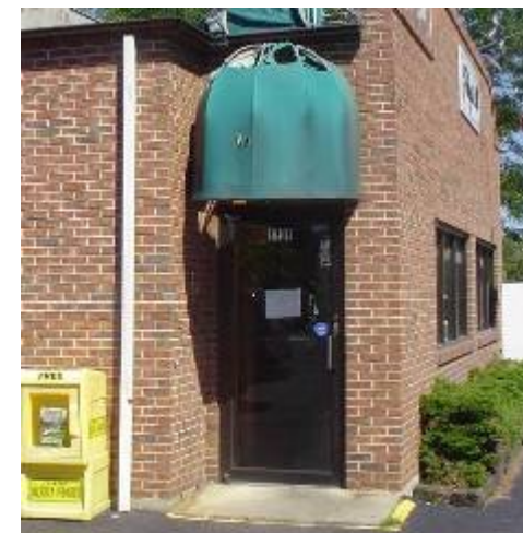
Awning is torn, frayed and soiled (3.4)
