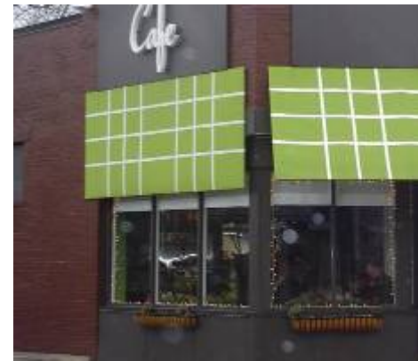
Awnings are not placed to provide weather protection (1b)
