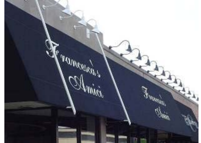
Gooseneck fixtures spaced too close together and too many in a row (4d)
